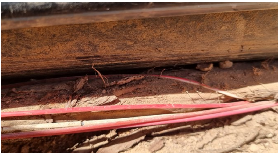
Figure 1: Existing cabling with tree roots.
